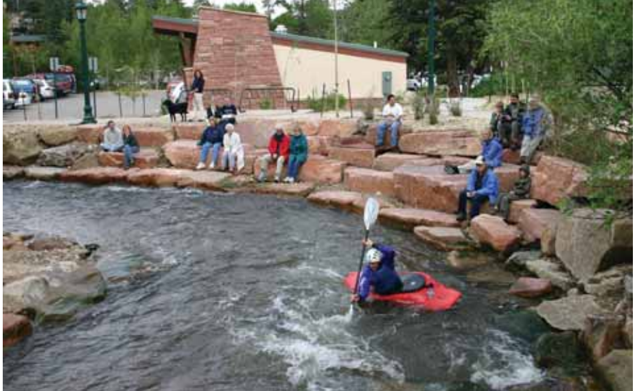
Where possible, existing boulders were incorporated into site-poured retaining walls along the riverbanks. Recreation and fish habitat were also considered. (Photo courtesy Design Studios West Inc.)
